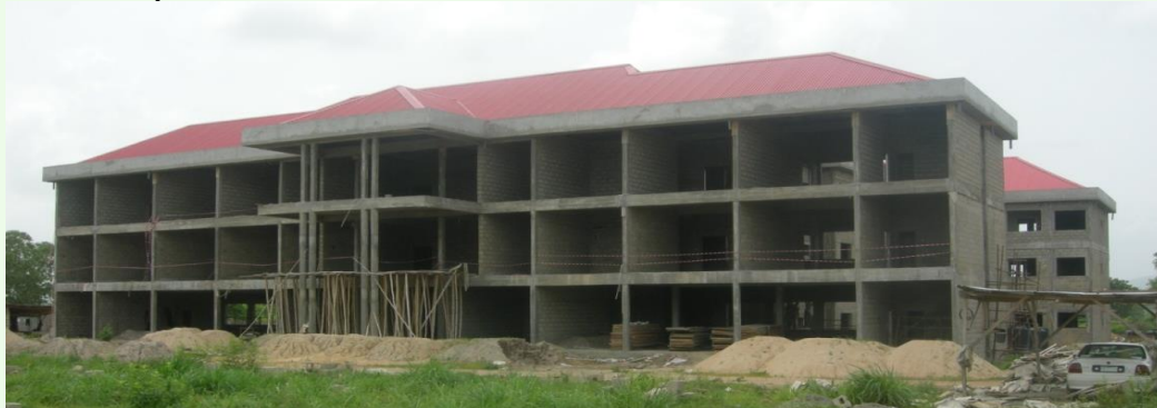
Figure 4a: The Multipurpose Research Infrastructure for Nuclear Instrumentation, Nuclear Safety and Nuclear Security Laboratories and Maintenance Workshops under construction at the NTC, Sheda, FCT.2015
