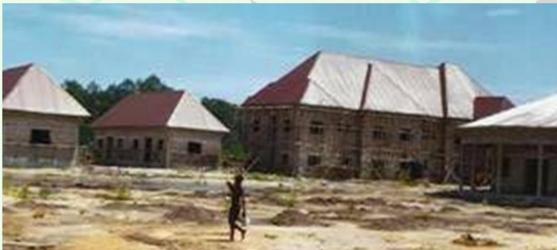
Figure 21: Physical and Research Infrastructure under construction at the FGN-IAEA Marine Contamination Coastal Field Monitoring Station, Koluama (2015)
